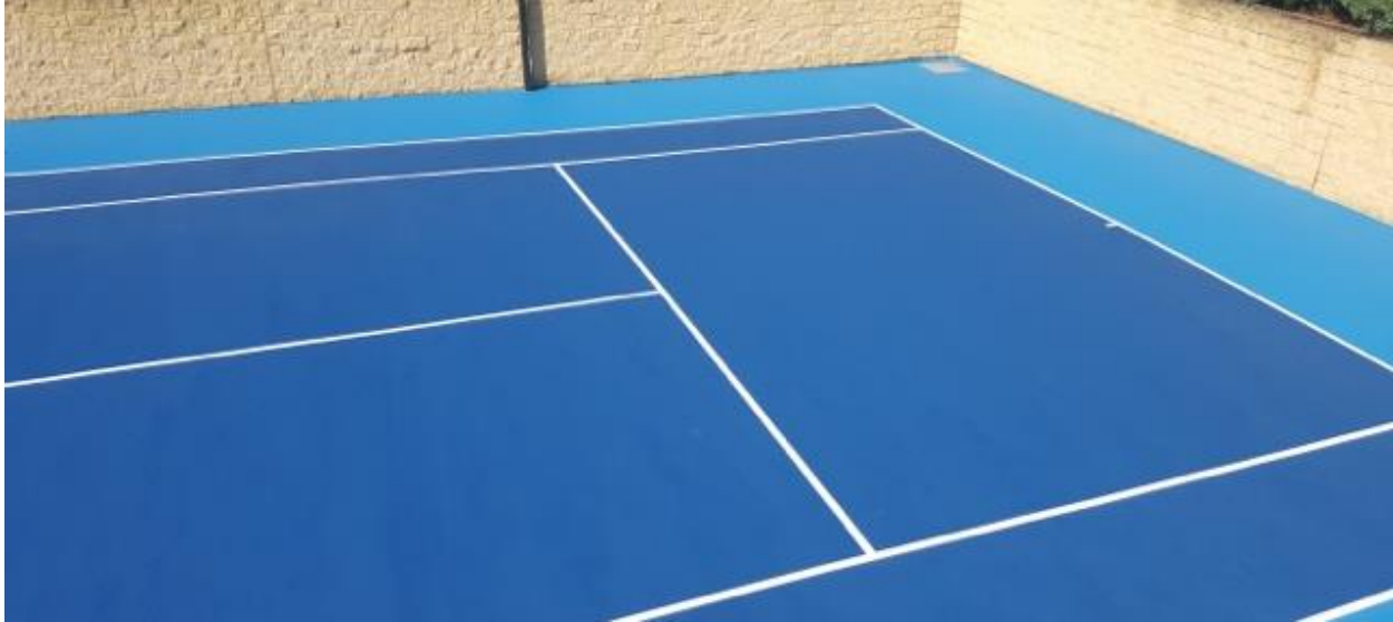
Catchment drain in corner of impervious court
