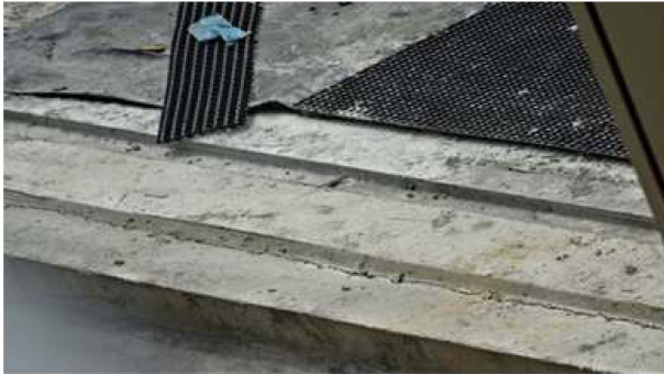
Photos: Poor Drainage Strategy has allowed the cork infill to float and move across the field due to the drainage cell not being deep enough and the collector drains at the edge of the field being inadequate for this type of rain event
